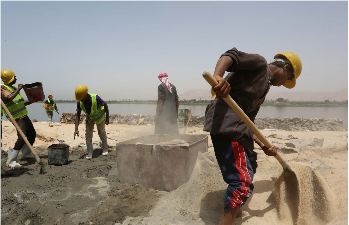
Workers build stronger banks on the Nile. Photo: © Dominic Chavez for World Bank.
