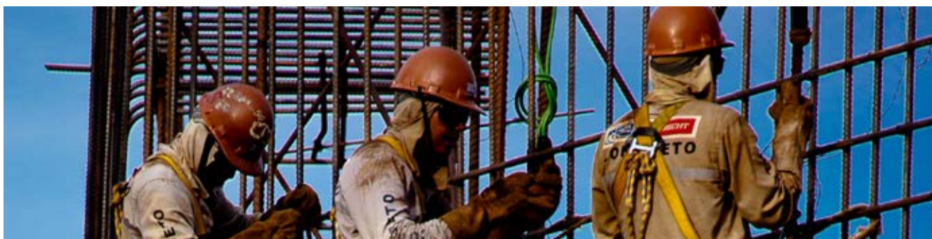
Works at the Santo Antônio hydroelectric plant at Porto Velho, Rondônia. Photo: © Divulgação Furnas
