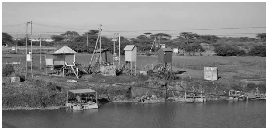
Pumps drawing irrigation water from the Awash River
