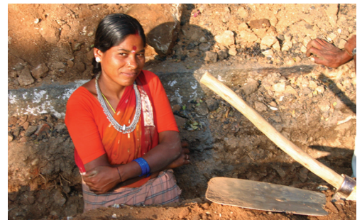
Woman digging a trench for a cable company in Hyderabad, India (Andy Hall)
